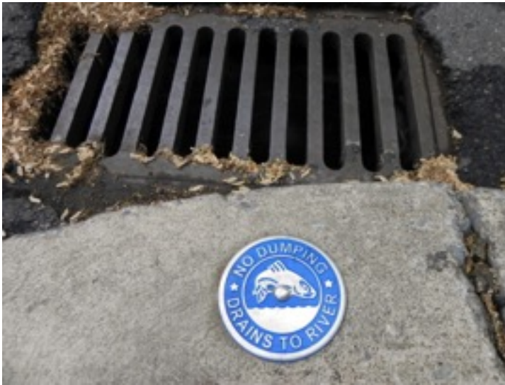
Photo of the top of a catch basin.
